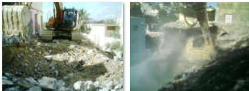
Photo 4-3: Demolition of Houses using Powered Mobile Plant in Phase I of the Project
