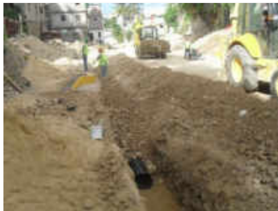
Photo 3-2: HDPE Pipeline installed in Phase I of the Project, similar to those to be used in Phase II
